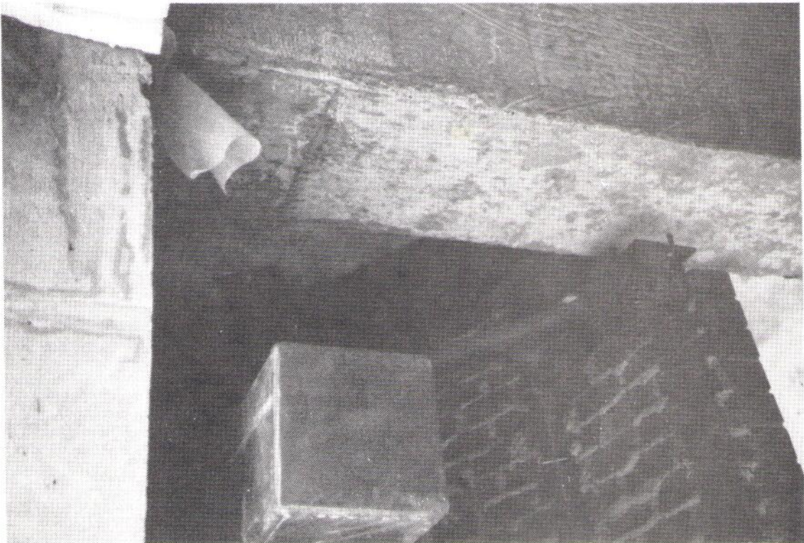
Photo 6: Detail of brick ties and fastening of prefabricated arch segment to the main structural elements
