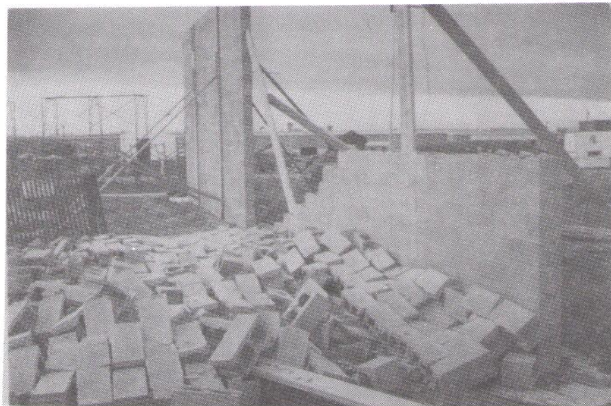
Photo 10. East Wall Blow Down.
